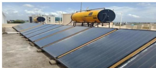
Solar Water Heating System
