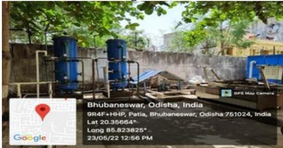
STP at Campus 18 (Capacity – 90 KLD)
