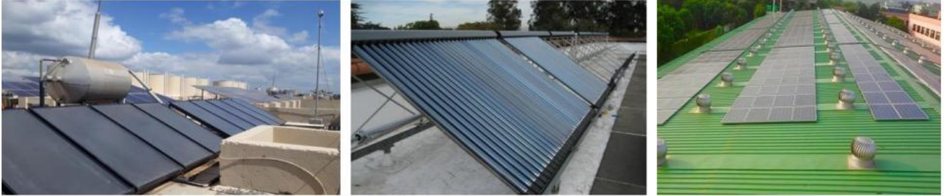
Solar Water Heating System
