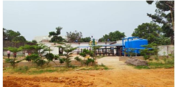
Sewage Treatment Plant at KIMS (2 million Liter per Day)
