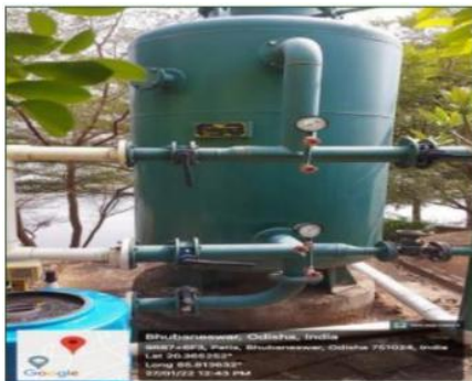
Liquid Waste Treatment Plants
