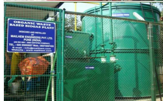
Fig. 7.3: Organic waste based Bio-gas generation plants placed at the campus
