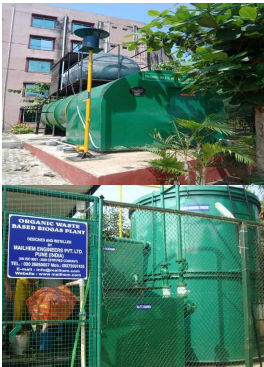
Fig. 13.2: Organic waste based Bio-gas generation plants placed at the campus
