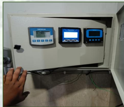
Figure 22. Water Quality Monitoring sensors.
