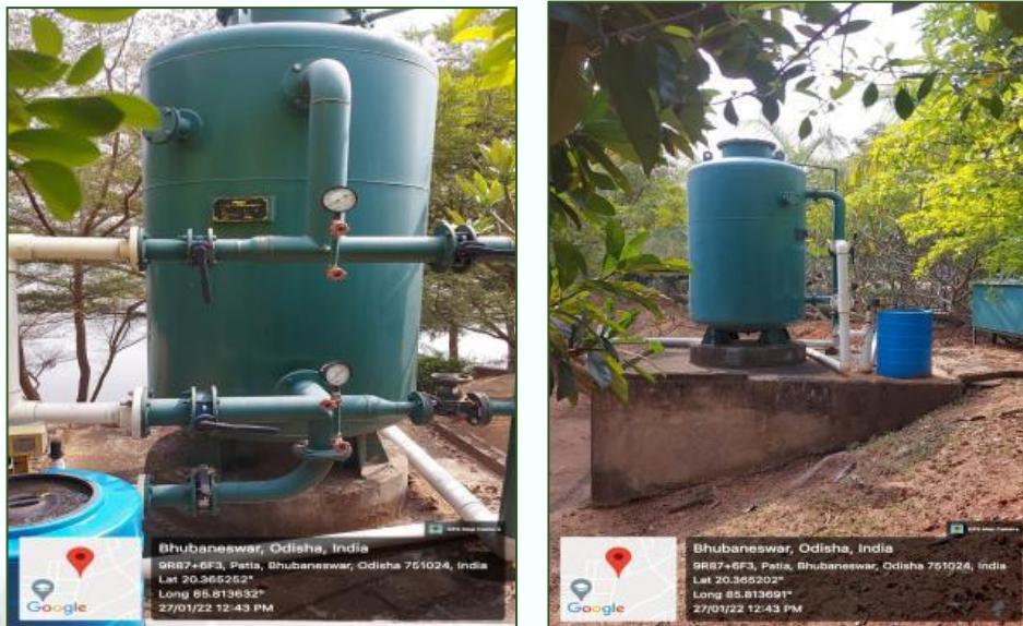
Figure 11. Liquid waste treatment plants.
