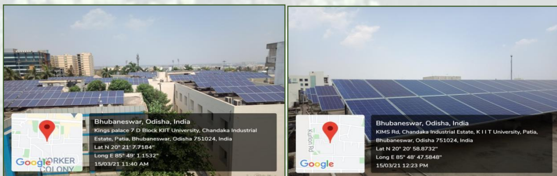
Figure 16. Solar PV rooftop systems installed over campus buildings.
