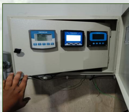
Figure 22. Water Quality Monitoring sensors.
