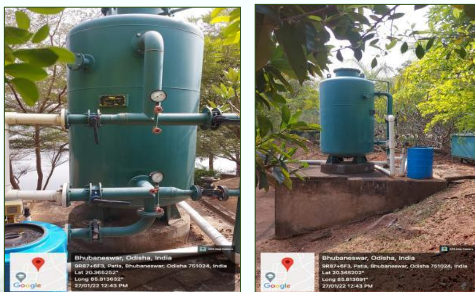
Figure 11. Liquid waste treatment plants.
